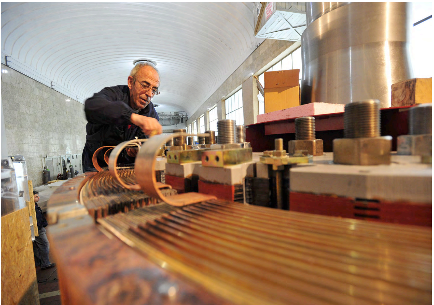
A man works on a generator at a Macedonia energy plant | © Tomislav Georgiev/World Bank
